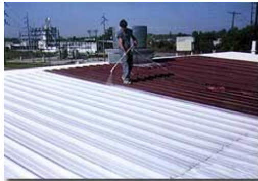
↑White coating for reflective roof [3]
