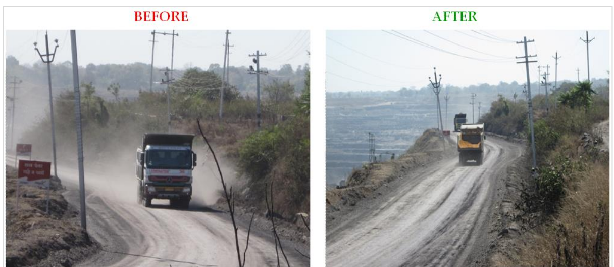
Figure 9: Case of Dustron PC Application in unpaved haul roads of coal mines
