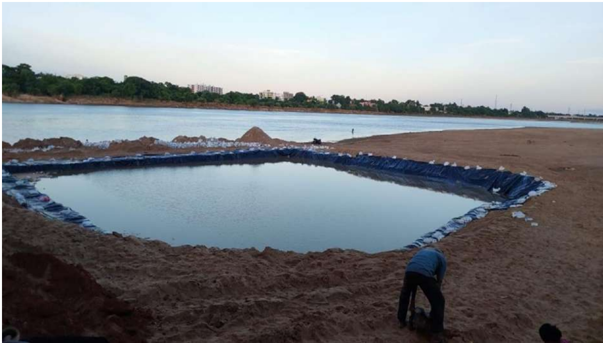
Fig. 2 Construction of temporary idol immersion pond on the bank of Kuakhai river in Bhubaneswar
