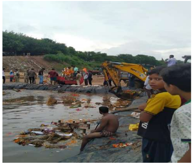
Fig.5 Removal of immersed left overs from the ponds to facilitate the immersion of other idols in the temporary immersion ponds
