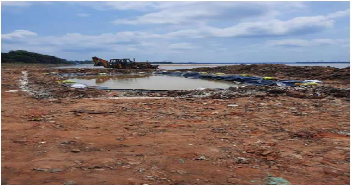
Fig.3 Construction of temporary immersion ponds on the bank of the Kathajodi river in Cuttack
