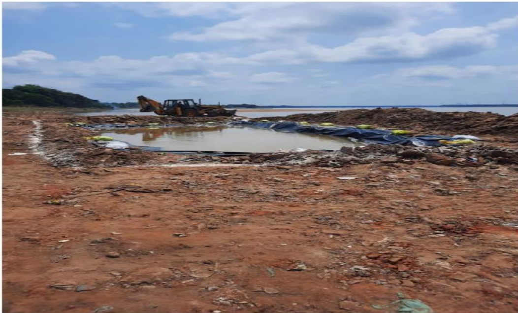
Fig.6 Construction of temporary immersion ponds on the bank of the Kathajodi river in Cuttack
