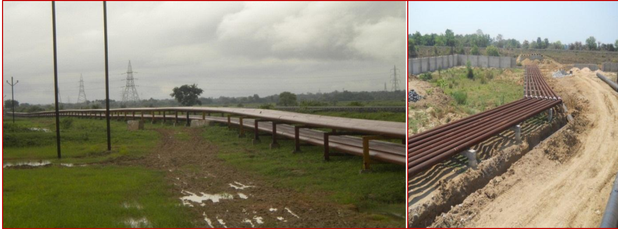
Slurry pipeline laid by NALCO (CPP), Angul for pumping lean slurry to Bharatpur Coal Mines
