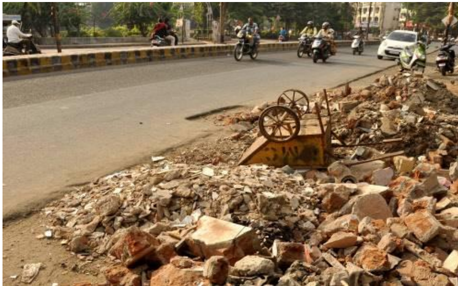
Figure 2.1: Indiscriminate dumping of C & D wastes along roadsides
